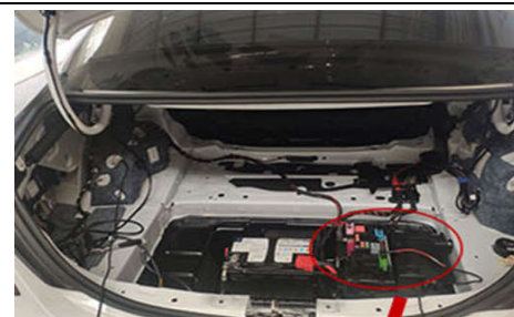
21. Get regular power in the fuse box
